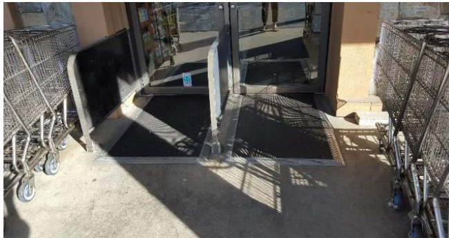
Example of pressure sensitive mats used at a market entrance/exit
