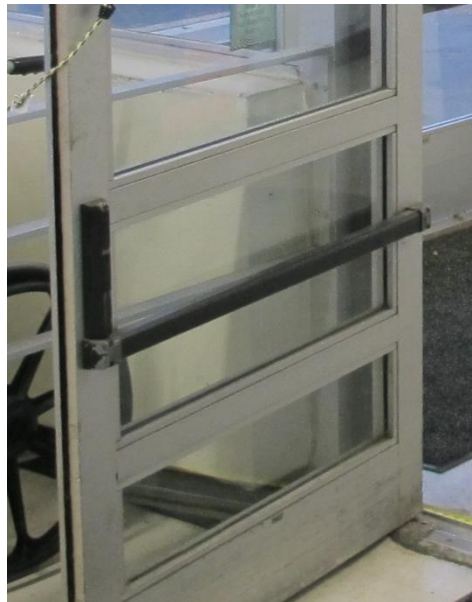
Swing door with older style presence detecting door mounted device
